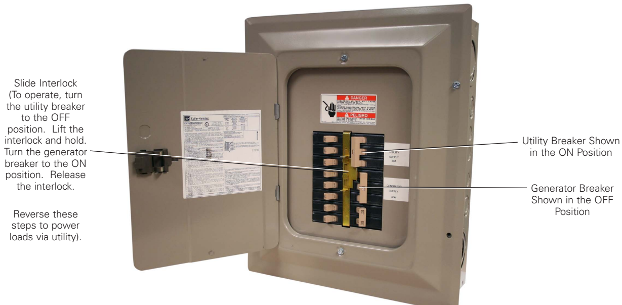
Figure 1. Manual Transfer Switch with Door Open.
